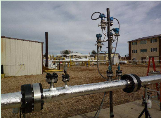
Wet Gas Venturi under FAT.
