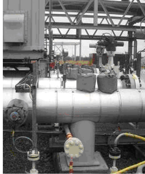
Fig 20. BP CATS downstream tap set up.
