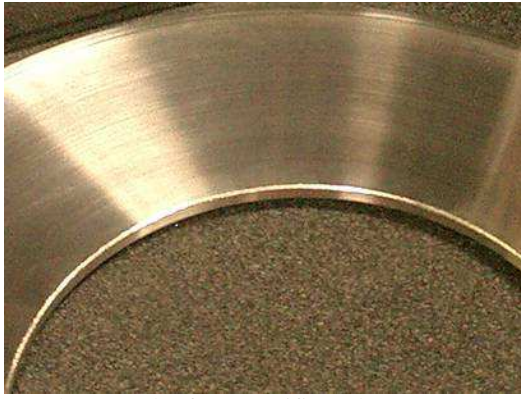
Fig 33. Photograph of worn orifice edge worn, 3 DP's.
