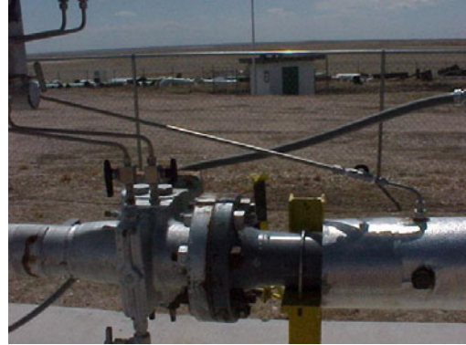
Fig 4. Orifice fitting with natural gas flow.
