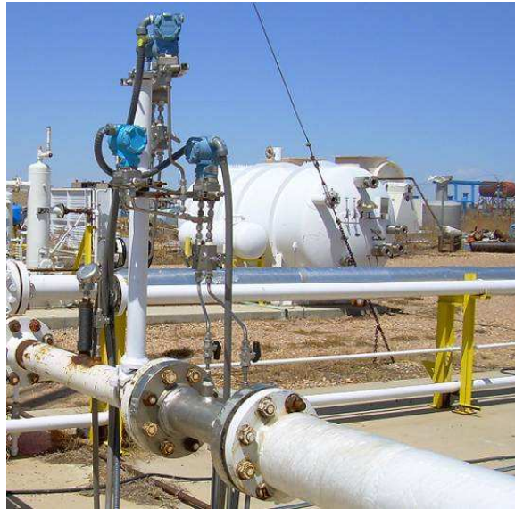
Fig 5. 4", 0.6 beta ratio Venturi meter installed in the CEESI wet natural gas loop.
