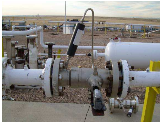
Fig 5. Close up of CEESI wet gas flow view port.
